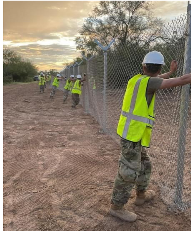
Exclusive photo of Texas National Guard fencing construction crew courtesy of Ken Oliver.
